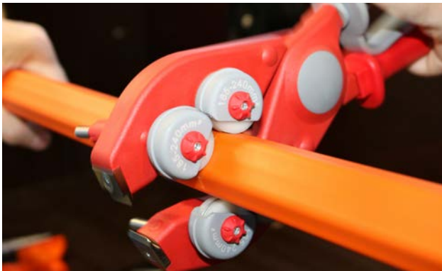
1. Notch the sheathing with the circular pliers at two spots at a distance of 60-100 cm from each other.
