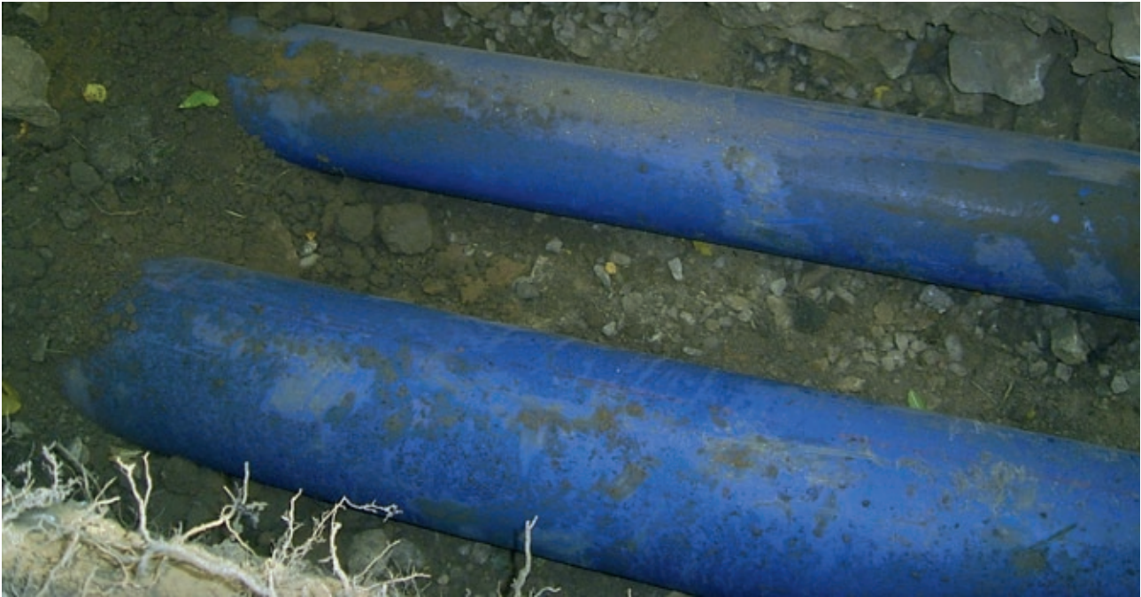
Fig. 17: PE pipes without protective sand bed
