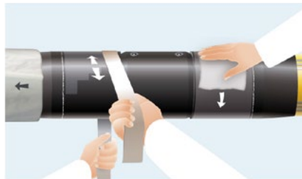
Fig. 2.14 Roughen the shrink area of the sleeve radially using emery cloth. Dry and clean the area subsequently
