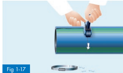
Fig 1-17 Removal of the protective layer with the egeplast M10 / M10 maxi peeling tool
