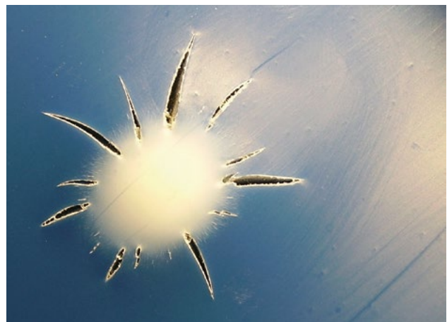
Fig. 19: Stress crack on the inside of the pipe caused by point load and incorrect choice of material (source: HESSEL technical engineering)
