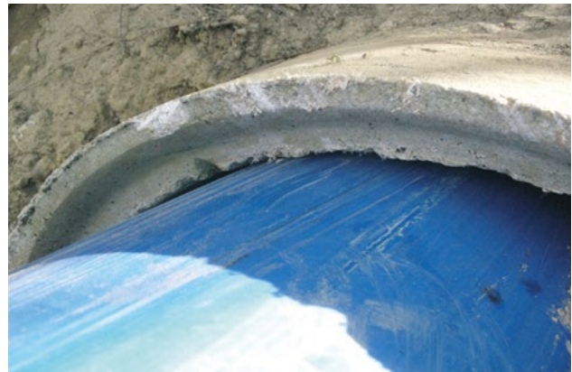
Fig. 13: Scratches and scoring arise during jacking that weaken the pipe wall and which therefore result in a curtailment in service life.
