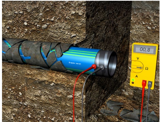
Fig. 25: Continuity check as evidence of lack of damage to the new pipeline
