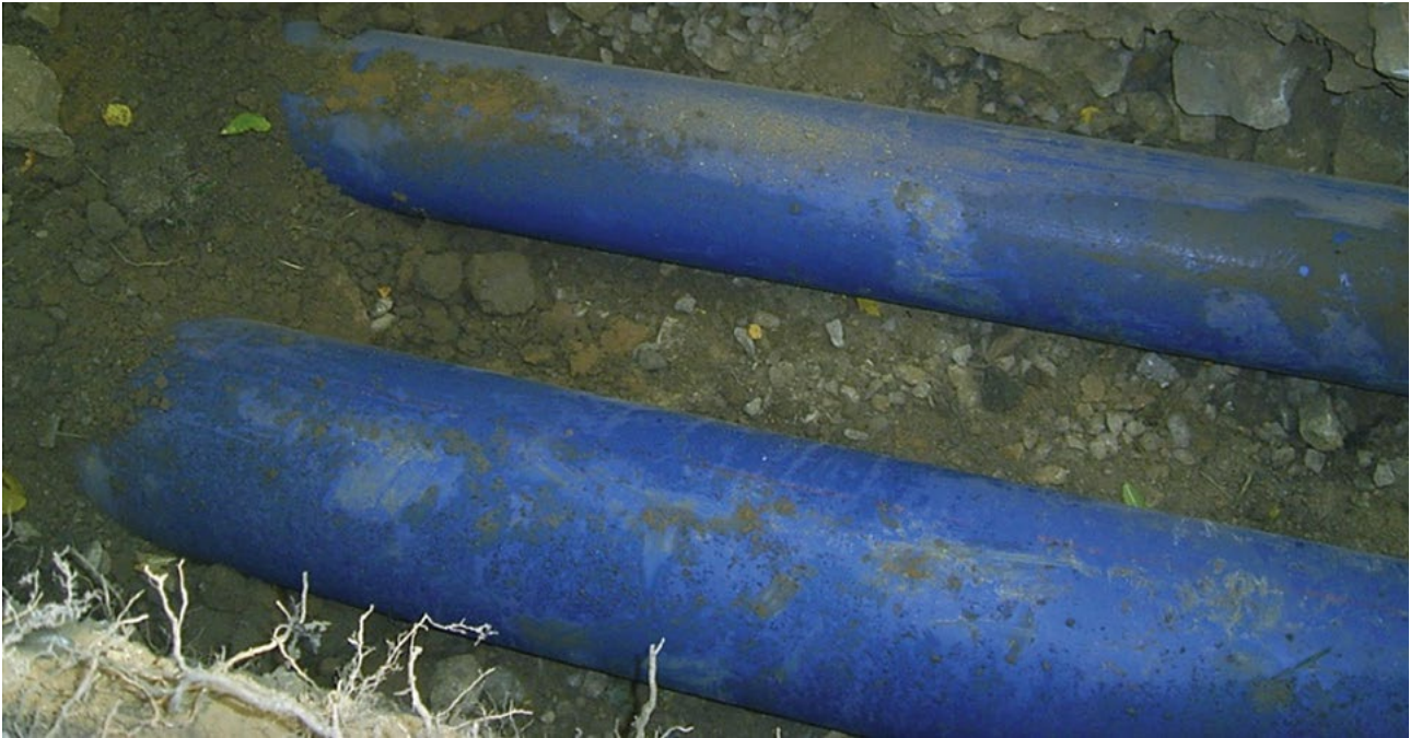
Fig. 17: PE pipes without protective sand bed
