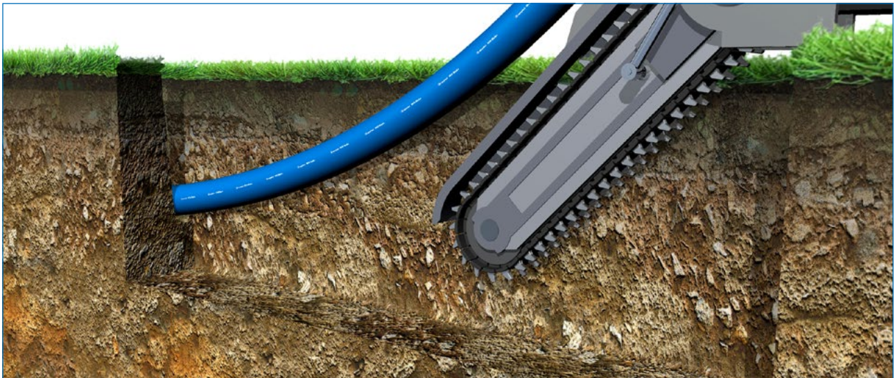
Fig. 6: Since excavated soil is used as backfill material in the milling method it is recommended that pipe systems with integrated protective layers be used.
