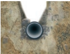
open trench installation without sandbed
