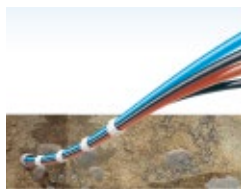
laying of pipe bundles with wastewater and potable water in one single route
