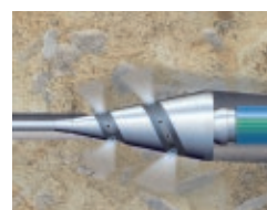
black-box installations such as horizontal directional drilling, bursting, relining and soil displacement
